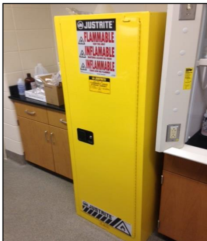
Figure 5.1 – Flammable Storage Cabinet
