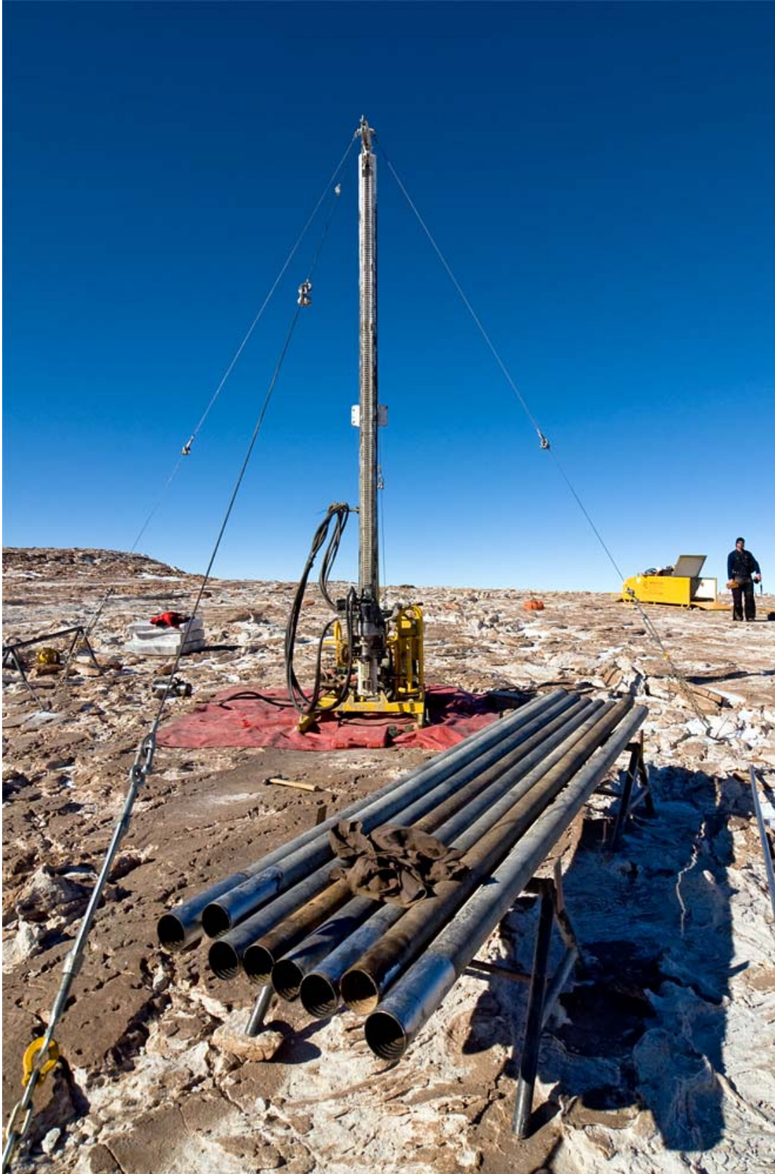
Rig and drill rods on Beacon Heights (before installing the shelter around the drill).
